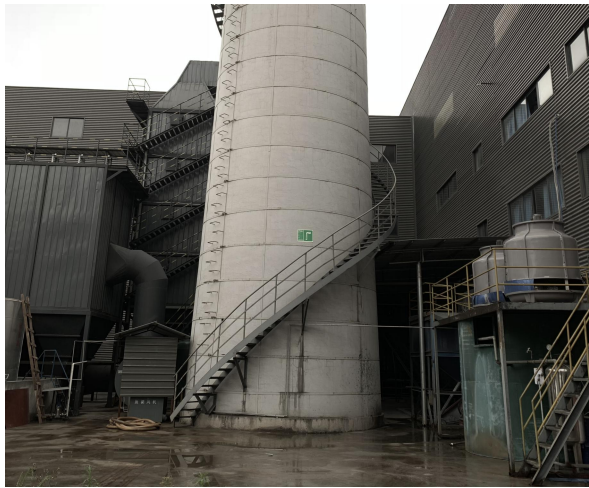
窑炉废气排气筒及标识
